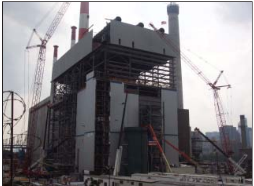
Proper noise control for Keyspan Energy's 250 MW Ravenswood Power Plant located in Queens, New York, U.S.A was challenging due to stringent local noise and structural stability ordinances. The combination power plant and compressor station incorporates a GE 7FA gas turbine and one steam turbine with HRSG.
